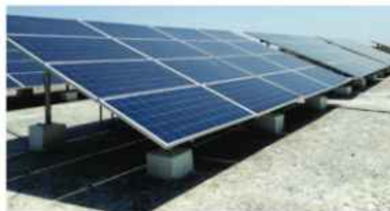
Solar Plant 100 KW
